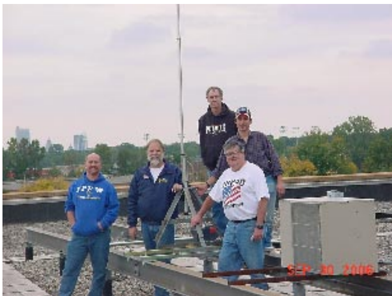
Installation of a new antenna on top of the Engineering Technology building for the IPFW Radio Station
